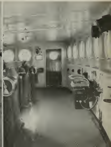
Transmitter-receiver installed in corner of chart room
